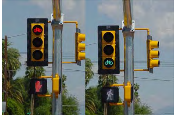
Figure 5.20 TOUCAN signal heads at North Stone Avenue and East Third Street
